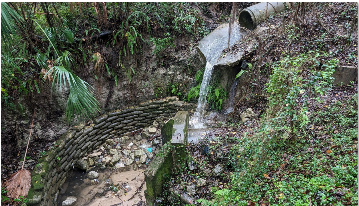
Figure 11. Graham Woods Erosion and Pipe Outlets
