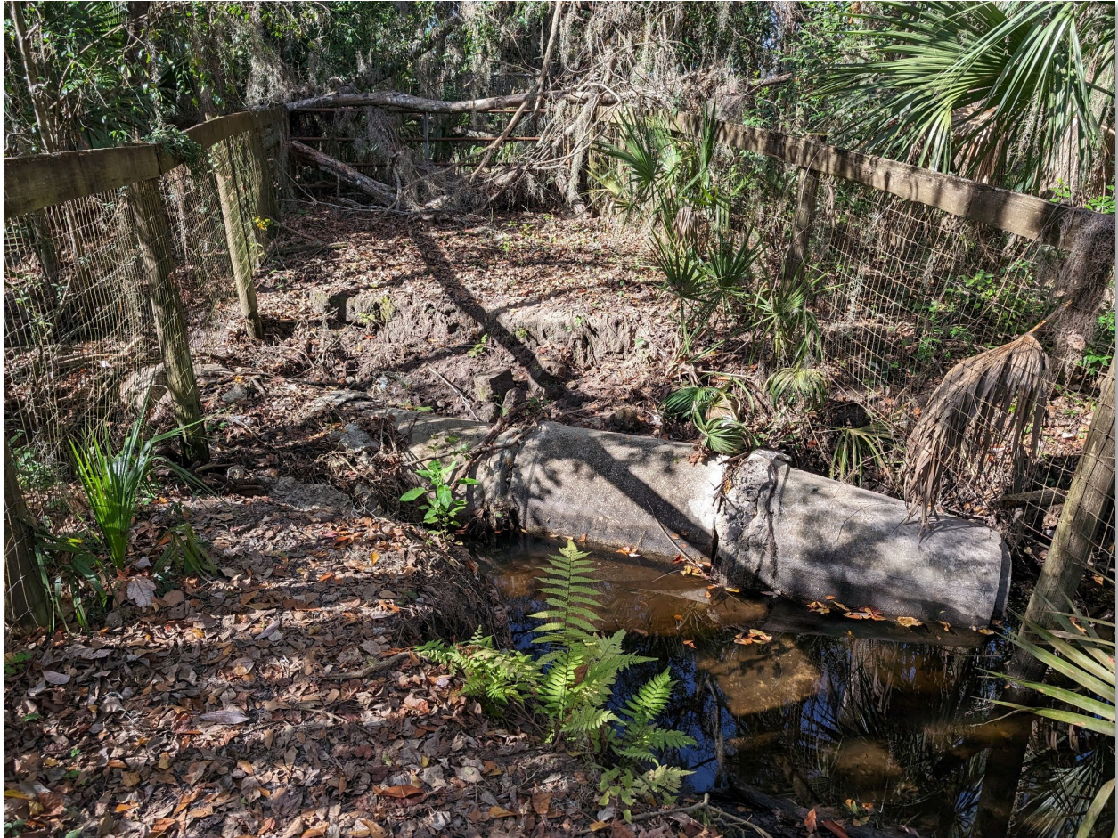
Figure 16. Washed-Out Dirt Road in Lake Alice South Conservation Area
