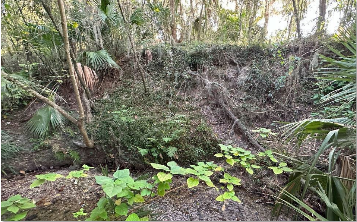
Figure 69. Erosion and Bank Failure in Reitz Ravine Woods
