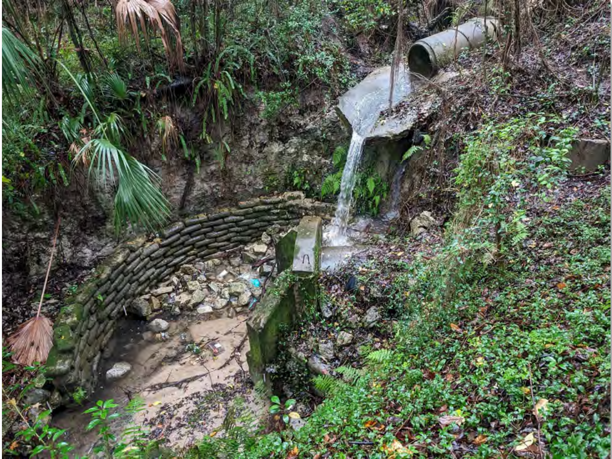
Figure 8. Graham Woods Erosion and Pipe Outlets
