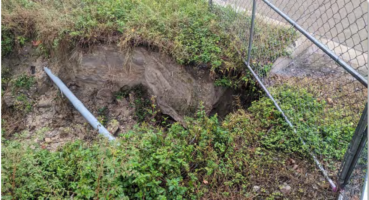
Figure 7. Keys Complex Erosion
