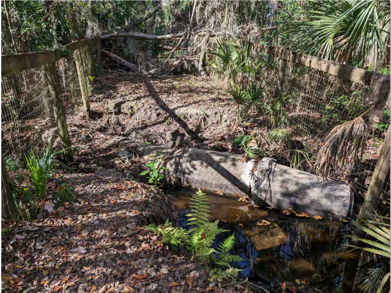
Figure 13. Washed-Out Dirt Road in Lake Alice South Conservation Area
