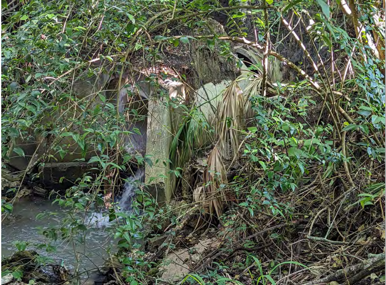
Figure 5. Jennings Creek Headwall Separation
