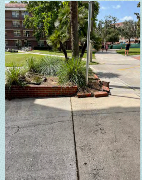
Broken Planter Wall
